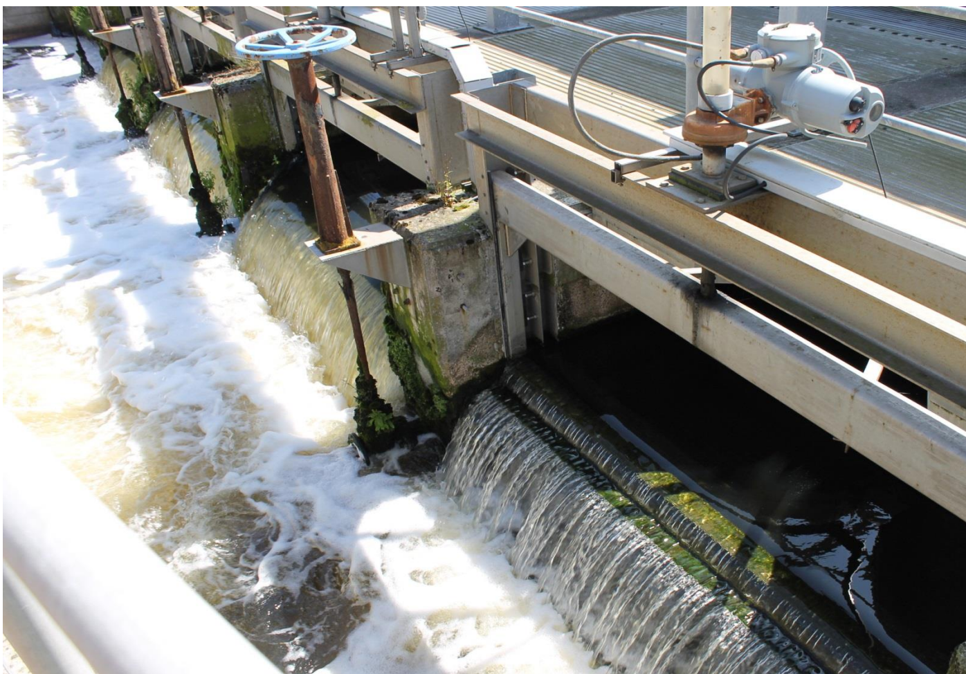
Photo : Seafield waste water treatment works, Scotland - Aqua Publica Europea
