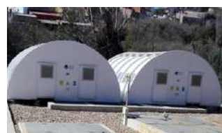
Rotating biological contactor
